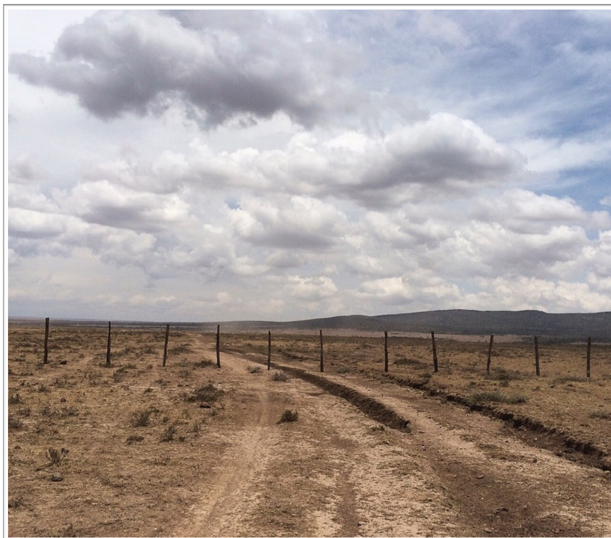
Loss of connectivity: Fencing newly subdivided plots with cedar posts sourced from Narok County's remaining forests now characterises the Loita plains.
