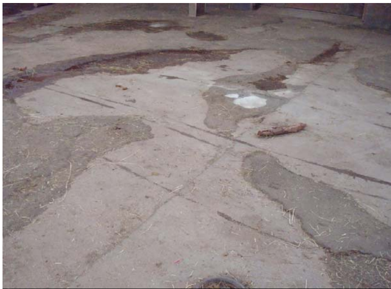
FIG. 9: REMINANTS OF RUBBERISED FLOORING LAID ON TOP OF CONCRETE
